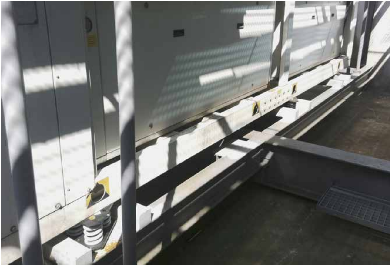
Ventilation system insulated with VIBRABSORBER
