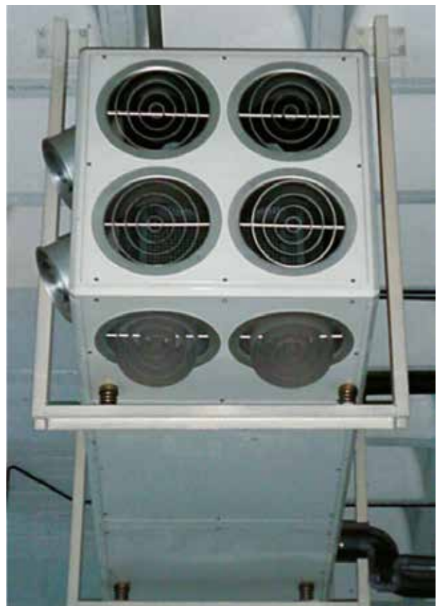
Ventilation system insulated with VIBRABSORBER®
