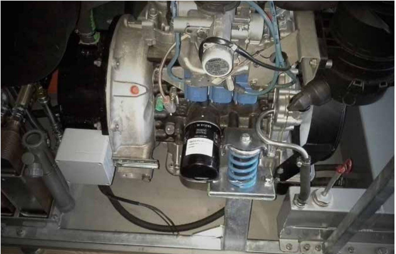
Generator set insulated with VIBRABSORBER+Sylomer®
